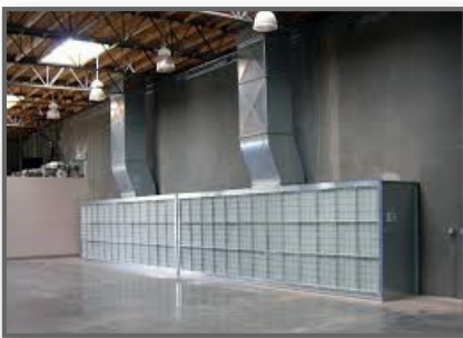
Air filtration rack
